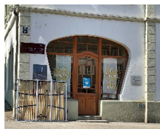
Non-respect de la structure architecturale.
